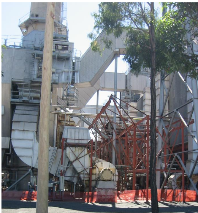
Callide-A Demonstration Plant, Queensland, Australia.
