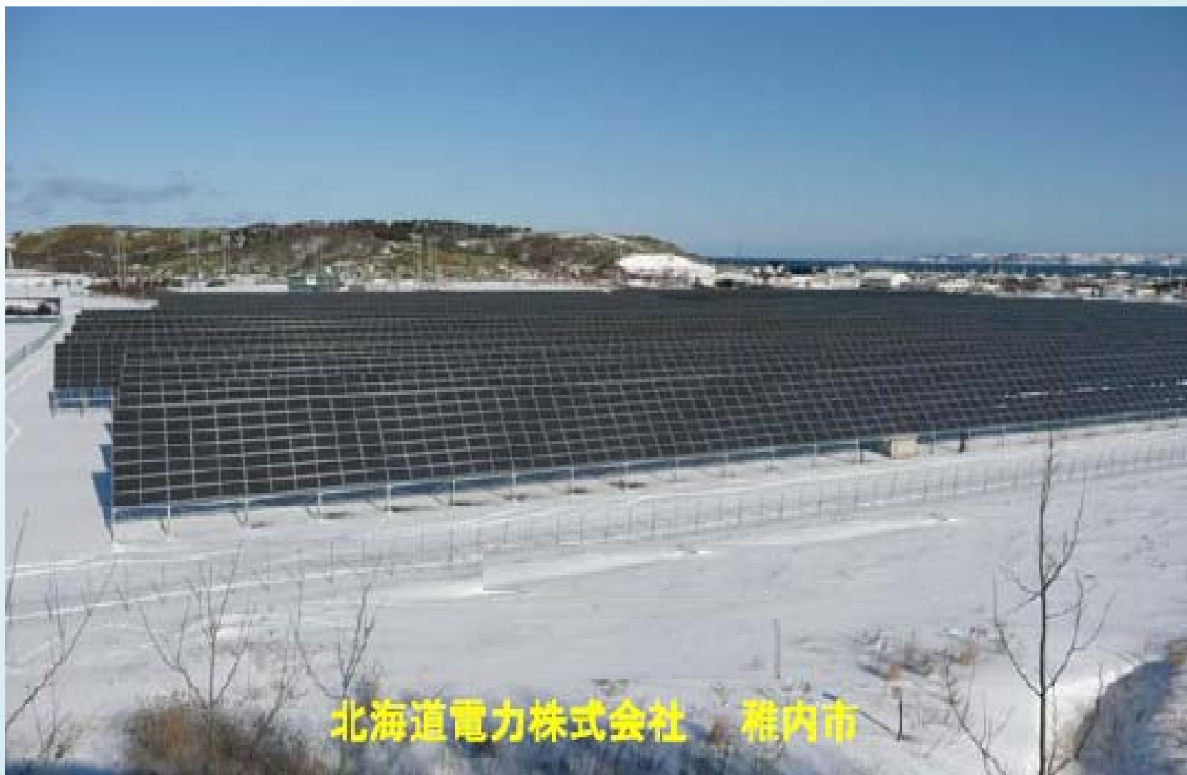
4MW Installation at Wakkanai site (Jan. 2009)
