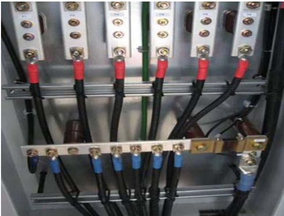
Main Combiner Box (MCB) Connection
