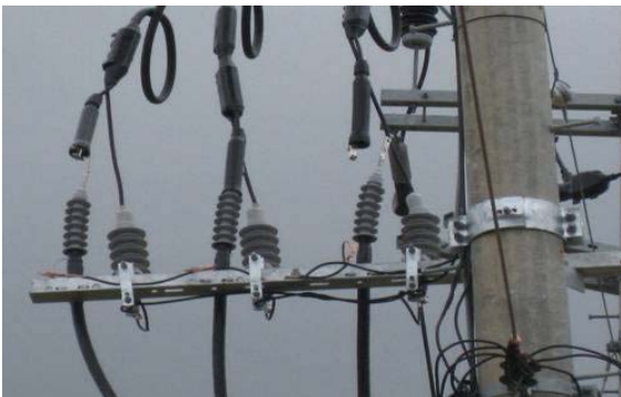
Electrical (22.9KV Cable connection) to Pole
