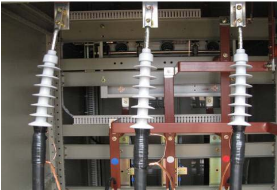
Electrical (22.9KV Cable connection) to Switchboard Panel
