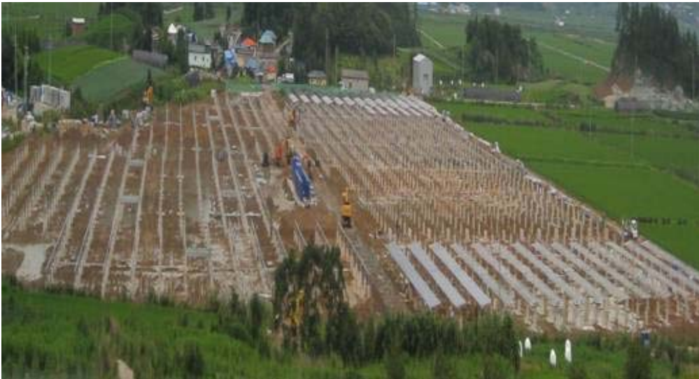
Panoramic view of the project site two thirds of way through construction (late Jul-09)
