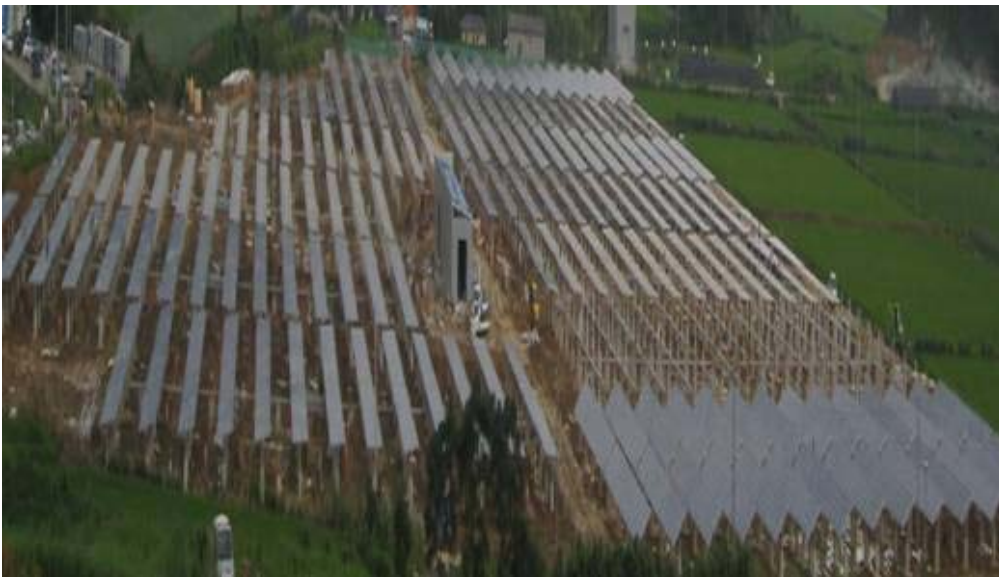
Panoramic view of the project site towards the end of construction (early Aug-09)
