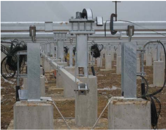
Installation of the tilt axis and linkage components of the tracking system
