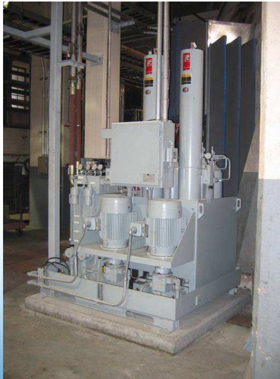
New Governor Oil Pumping Unit
