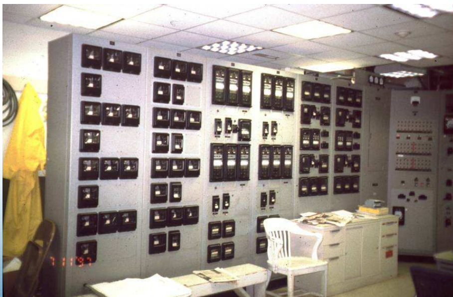
Old Electromechanical Relays
