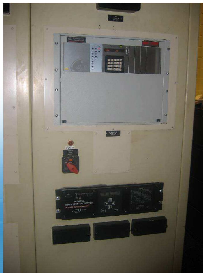
Modern Multifunction Microprocessor Relays
