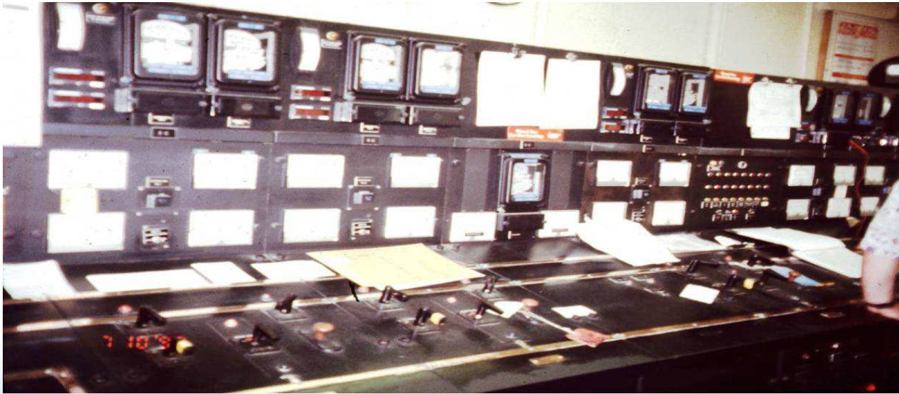
Old control boards
