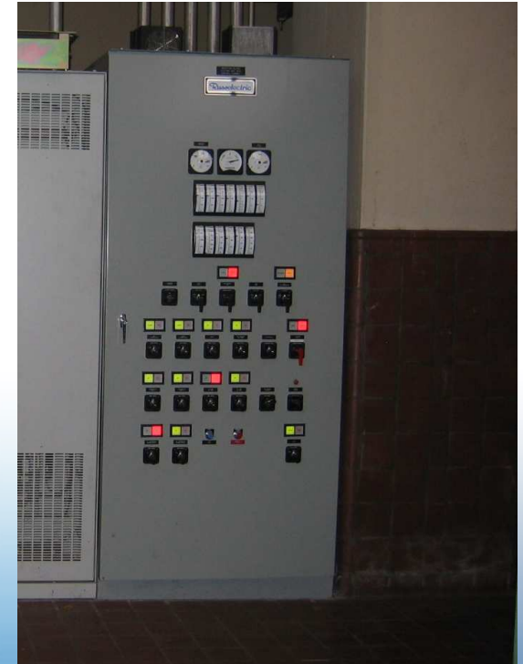
Unit Control Cabinet (Programmable Logic Controller incorporates all unit control as well as governor logic)
